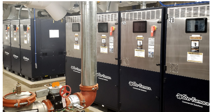
WaterFurnace’s TruClimate 500 modular chillers have helped CSU Moby Arena cut its energy usage by 50%.
